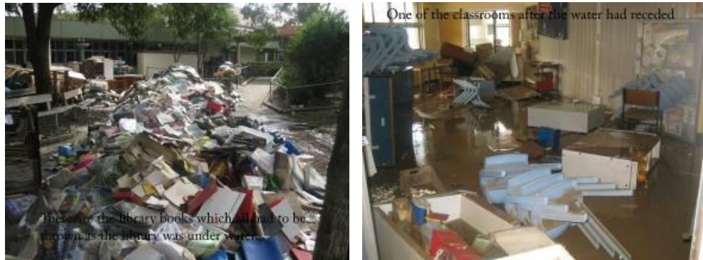
Flood damaged schools in Queensland, Australia
